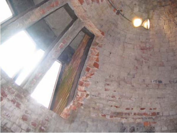
View looking up at the "cut away" viewing glass.
