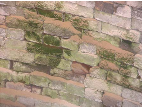
Plant growth on the interior brick.
